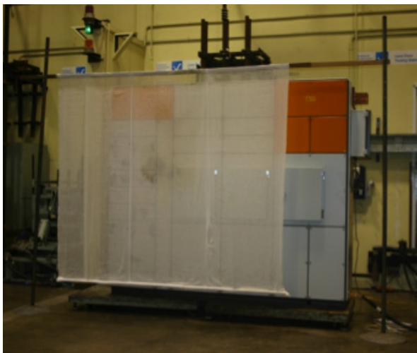
Figure 8: A CUBIC switchboard undergoing arc fault containment testing.
