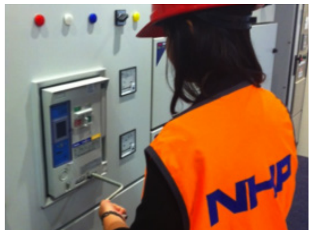
Figure 6: A maintenance worker manually racks the ACB from the connected to the isolated position.
