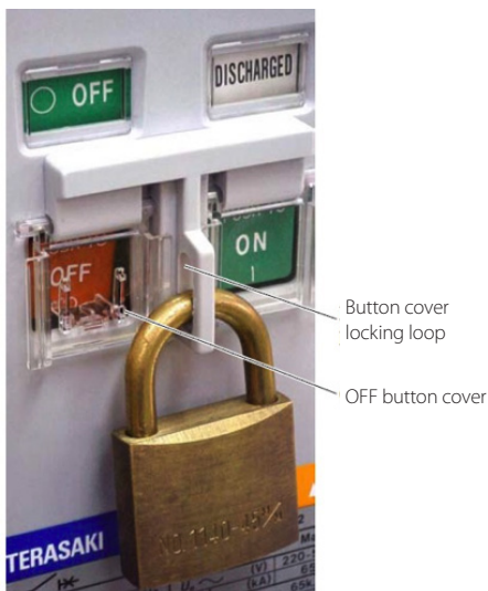
Figure 1: Using a padlock to lock off an air circuit breaker (ACB)
