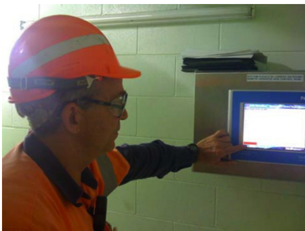
Figure 5: A site engineer uses a HMI to view the status of the ACBs in the adjoining switch room.
