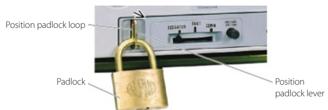
Figure 3: Using a padlock to lock an ACB in the ISOLATED position
