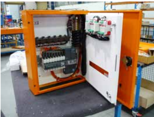
ATyS M installed into a panel board
