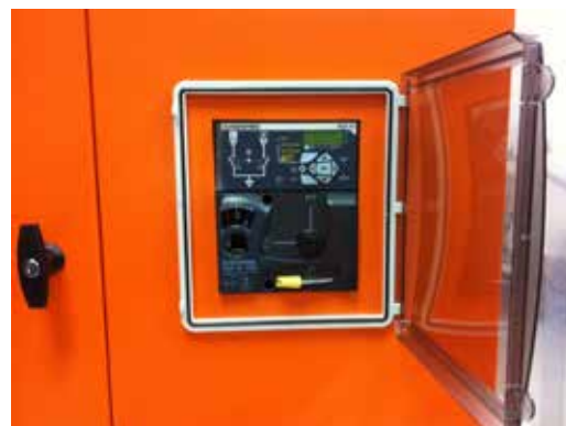
Main Switchboard mounted ATyS
